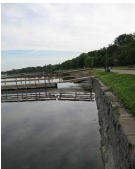
WPA walls are in need of restoration.
