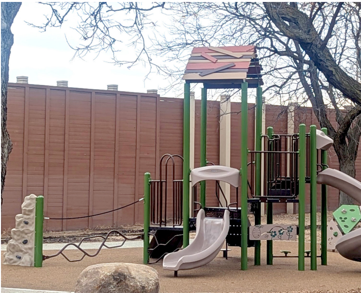
Construction at the 28th Street Totlot began in the fall, with a new playground, entry plaza and path, site furnishings and landscaping to open in 2025.
