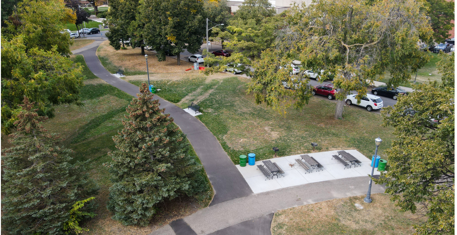
Summer construction at Murphy Square Park improved access and circulation by changing paths, lighting and locations of site furnishings.
