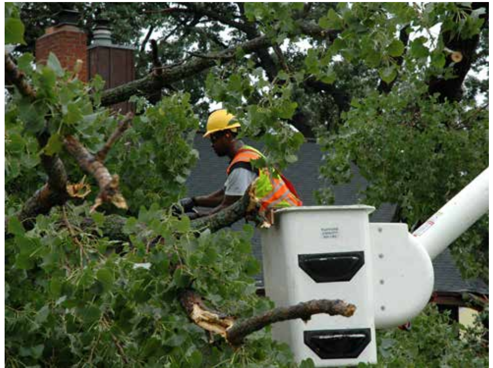
Figure 89. Tree removal following storm damage.
