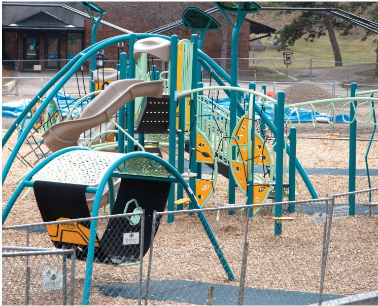
Construction of major improvements at Sibley Park (above and top) began in spring; a new playground with a zipline opened by the end of the year, while the ADA-accessible wading pool is planned to open by summer 2024.
