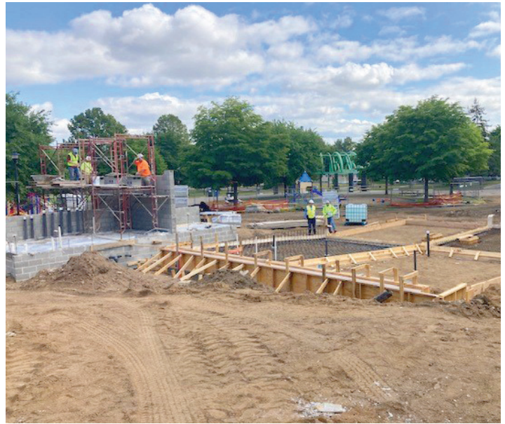
Construction proceeded throughout the season on Jordan Park's accessible wading pool with splash features, along with a restroom building, fencing, various amenities, and lighting upgrades throughout the park. This project will be complete in 2024.
