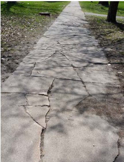
Trails in poor condition
