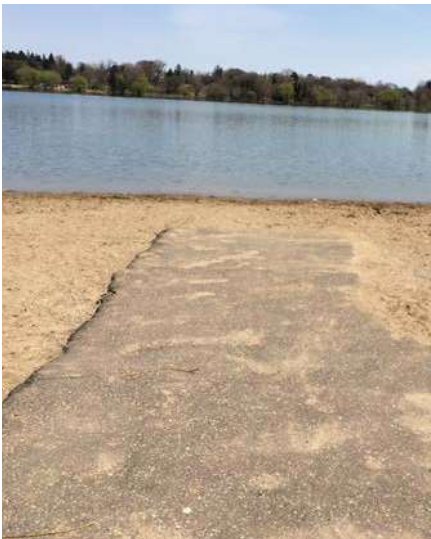
The master plan proposes a fully ADA accessible pathway to the lake.
