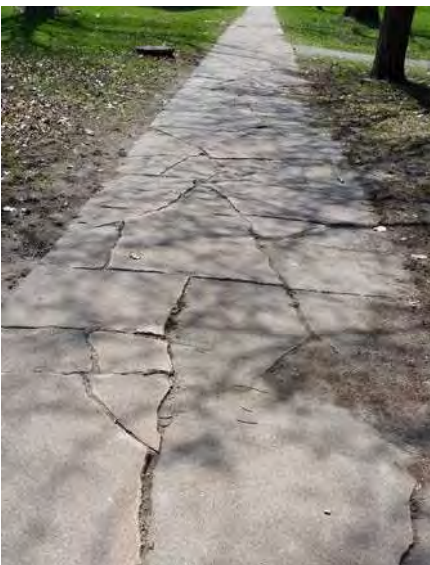
Trails in poor condition
