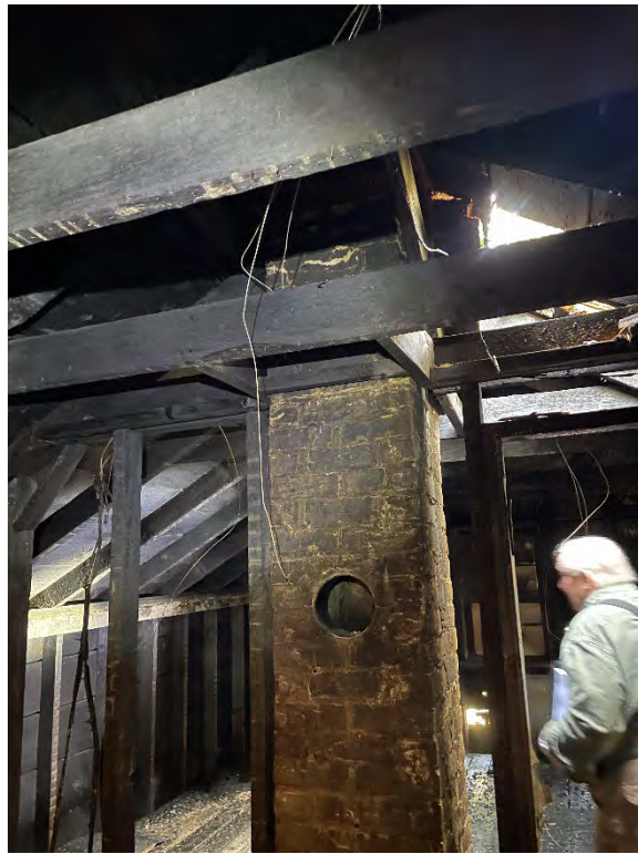
Photo 35 South chamber chimney condition.
