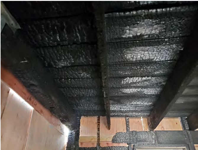
View within the first floor near the northeast corner illustrating the damage to the wall and second floor framing.
