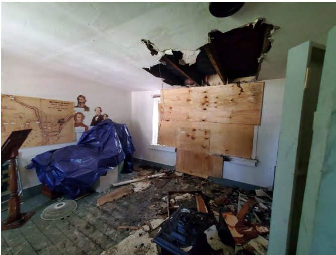
View at the first floor within the two-story section after the second fire. Damage was limited to several of the east wall studs and approximately three second floor joists.
