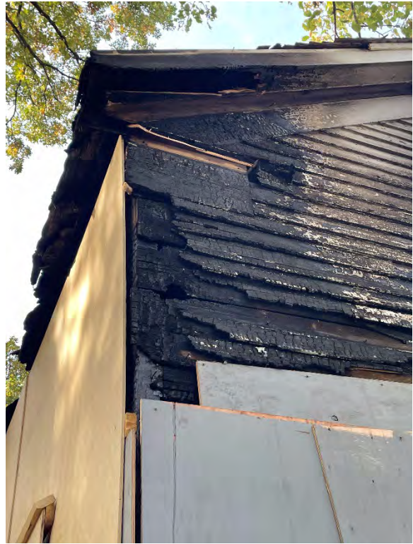
Photo 15 Closeup of damage on NE corner.
