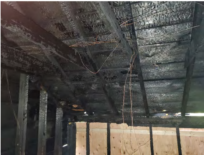
View within the second floor near the northeast corner illustrating the damage to the wall and roof framing. Nearly all of the roof framing and roof sheathing was affected. The wall studs at the east and north walls were also severely damaged.
