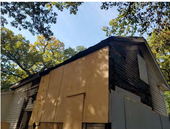
View from the northeast corner after the third fire. This fire has damaged a considerable portion of the north half of the two-story section.
