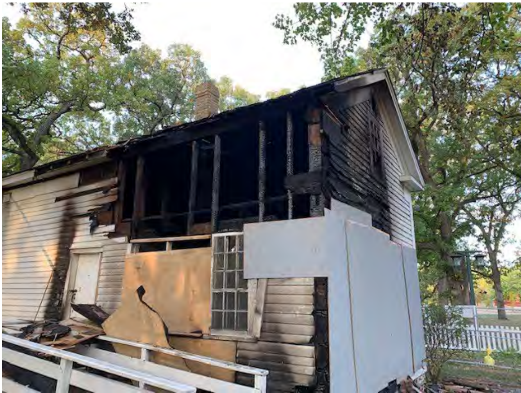
Photo 36 After third fire before plywood installation.
