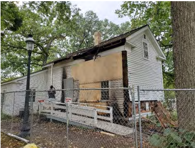
View from the northeast corner. The fires have originated near this corner. This photo is after the second fire event.
