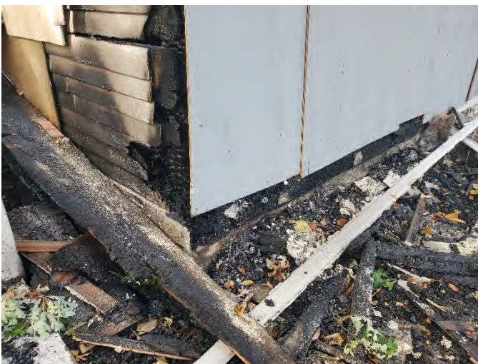
The fire has damaged the timber sill at the base of the walls but the first-floor framing, basement and foundations have been relatively unaffected.
