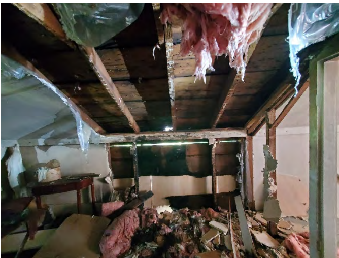
View of the second floor and roof framing within the two-story section after the second fire. Fire damage affected only the roof eave and east wall studs. The roof framing was relatively unharmed.
