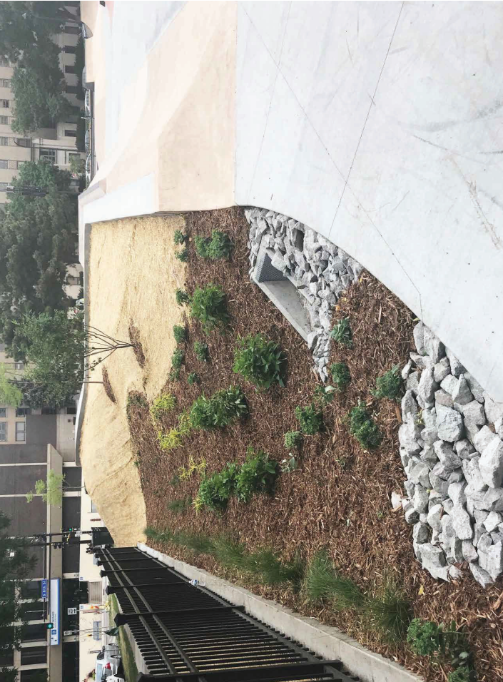
Stormwater Treatment Swale
