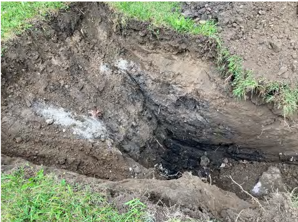
Photo 8: TE-05-20, north end, exposed footing
